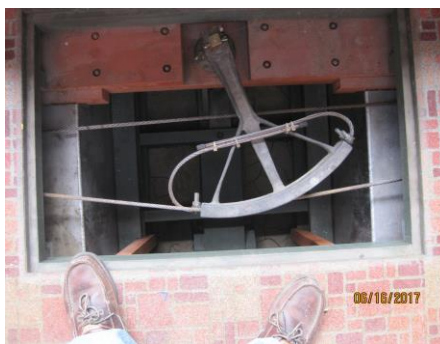
Steering Cable loose at Quadrant
